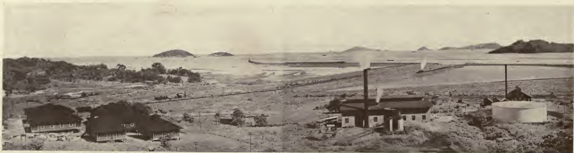
Overlooking the Pacific, showing the canal entrance, and Naos and Flamenco Islands in the distance. The Naos Island breakwater under construction. The Pacific entrance requires no protection from storms, but the breakwater is to prevent shoaling of the channel. Land at the inner end of the breakwater is being reclaimed for a townsite and other purposes. Over 300 acres have been filled in with spoil excavated from the canal prism.
